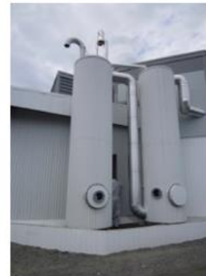
Ozone contact towers
